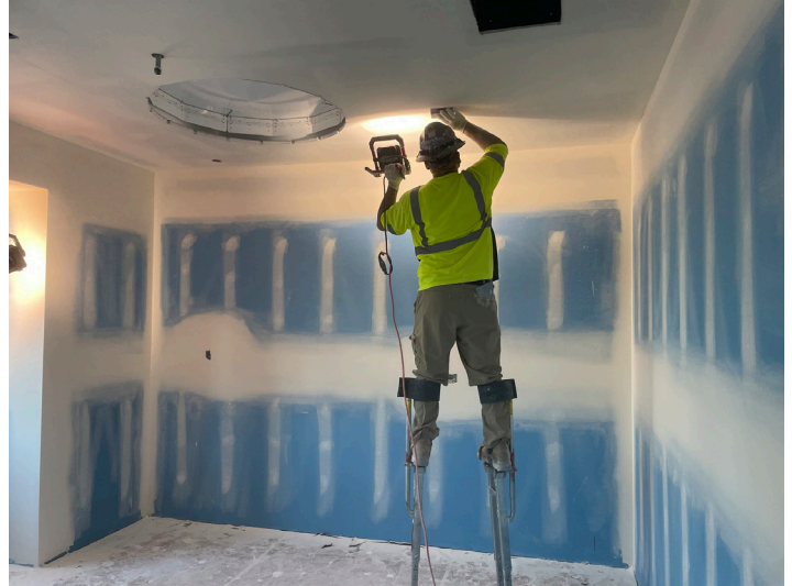
DWI taping and finishing the sheet rock in prep for paint in residential inpatient.
